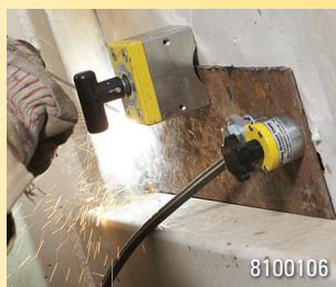
Helping hand – a temporary support to hold a part or tool on a vertical wall.
